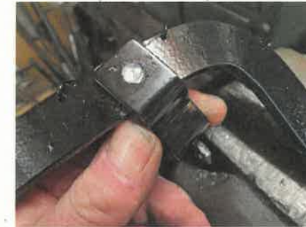
12 First job was remove rear brackets; they reach too far forward. Pruning them back will move the saddle nose forward and closer to the frame lug.
